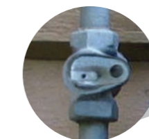
Closed gas meter valve
