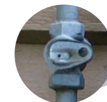
Closed gas meter valve
