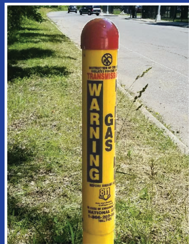
Natural gas pipeline markers are generally yellow and black. They're placed near pipelines but not necessarily directly on top of them.
