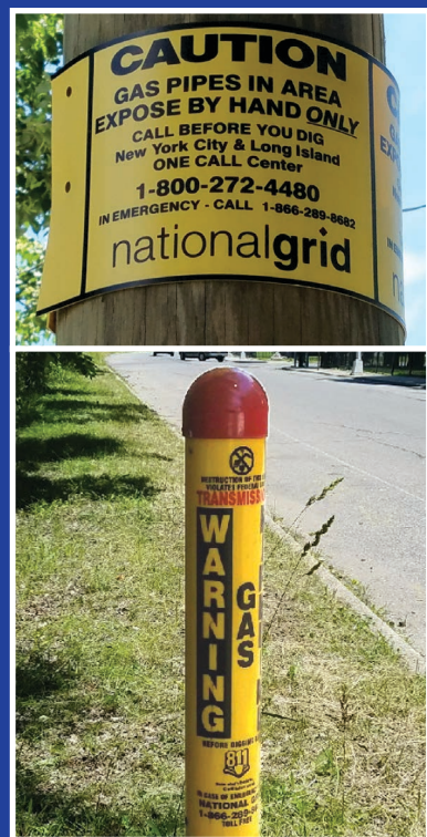
Natural gas pipeline markers are generally yellow and black. They're placed near pipelines but not necessarily directly on top of them.
