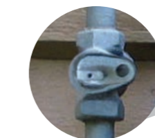
Closed gas meter valve
