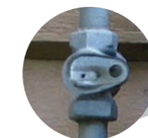
Closed gas meter valve
