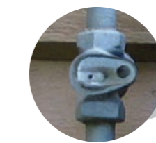
Closed gas meter valve
