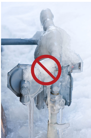
Never risk damage to natural gas equipment by kicking or striking it to remove accumulated ice or snow.
