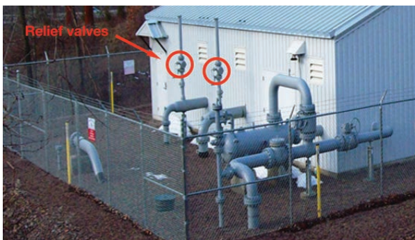
Dedicated relief valves are typically present in high-pressure distribution stations and at pressured storage locations.
