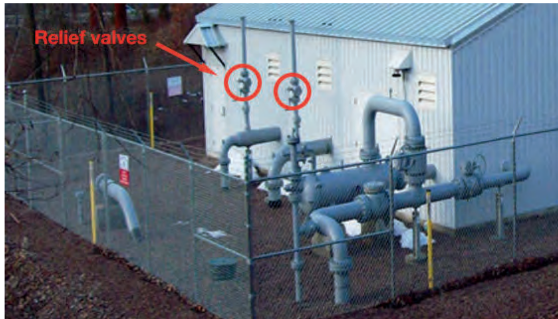
Dedicated relief valves are typically present in high-pressure distribution stations and at pressured storage locations.
