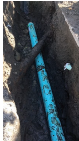
This excavation has encroached upon a cast iron natural gas main, exposing the gas main to potential damage.
