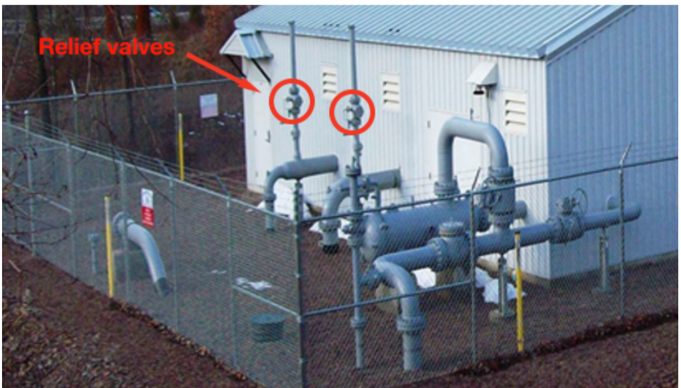
Dedicated relief valves are typically present in high-pressure distribution stations and at pressurized storage locations.
