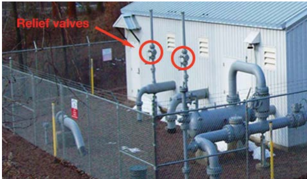
Dedicated relief valves are typically present in high-pressure distribution stations and at pressurized storage locations.
