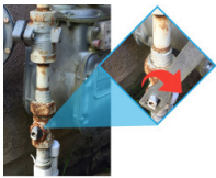
A gas valve is off when it aligns across the pipe.
